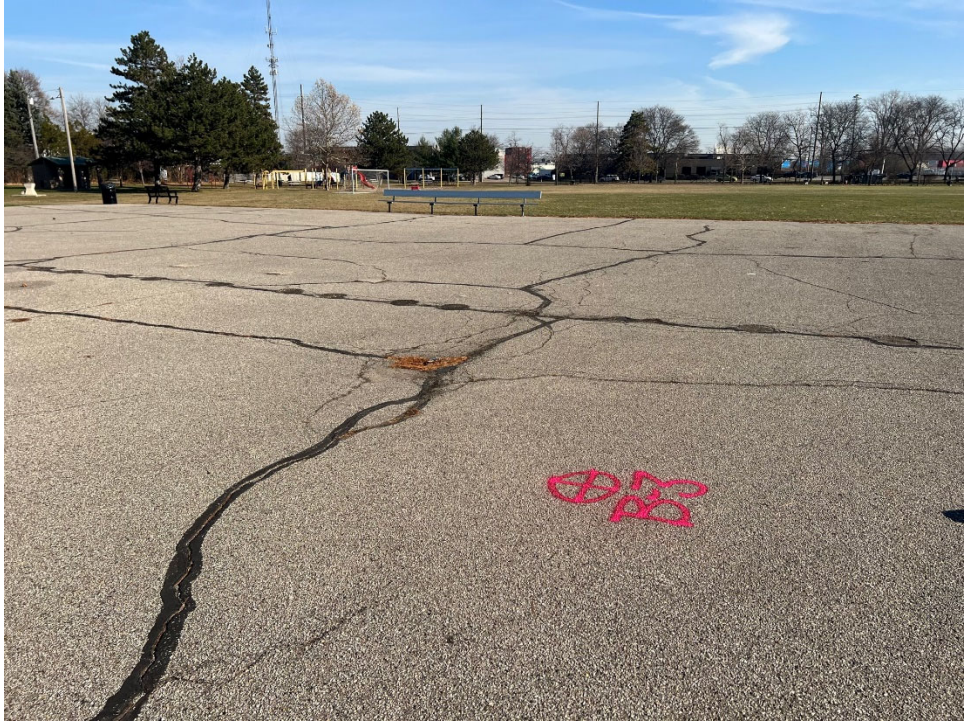
Photograph No. 3: Moderate to high severity transverse, longitudinal, block and fatigue cracking within existing pavements near boring B-03. View to the northeast.
