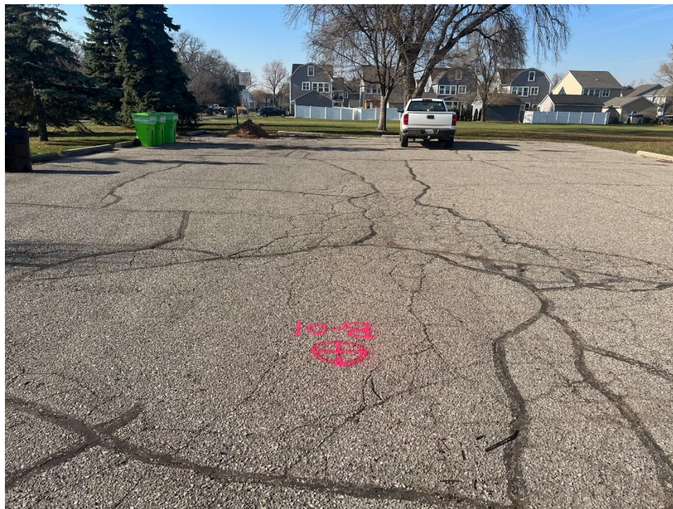
Photograph No. 2: Moderate to high severity transversal, longitudinal cracking within existing parking lot near boring B-01. View to the west.
