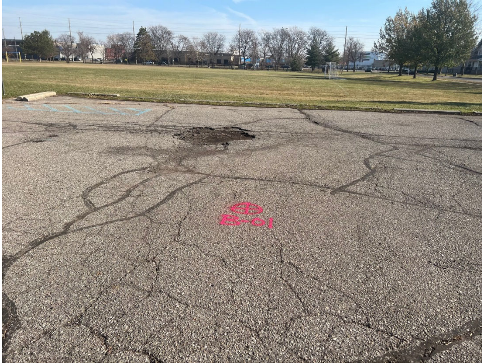
Photograph No. 1: Moderate to high severity transversal, longitudinal, block, and fatigue cracking within parking lot near boring B-01. View to the east.
