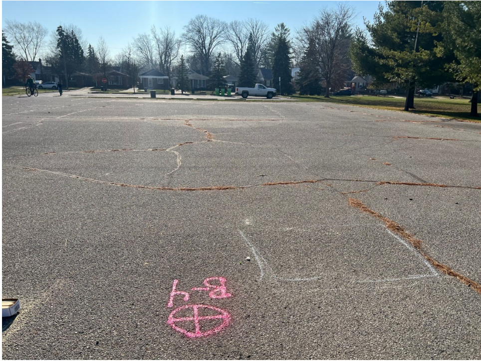
Photograph No. 4: Moderate to High severity longitudinal and transverse cracking within existing pavements near boring B-04. View to the south.
